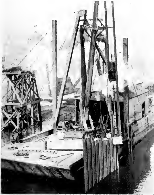
Driving 40 ft. Lackawanna arched web steel sheet piling to grade 20 ft. below extreme low water with 8,000 lb. steam hammer.
